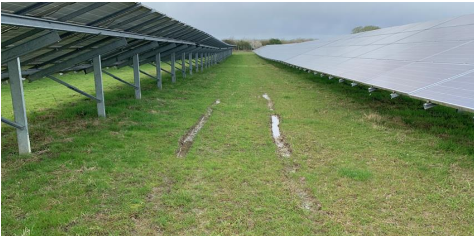
Insert 45: Ruts Caused by Vehicles
